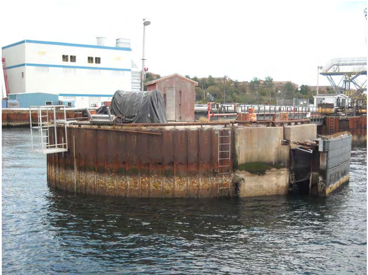
Typical SSP Condition in Tidal Zone Picture Taken at Low Tide
