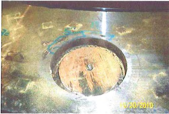
HOLE #19 WITH 5" LINEAR INDICATION AROUND HOLE
