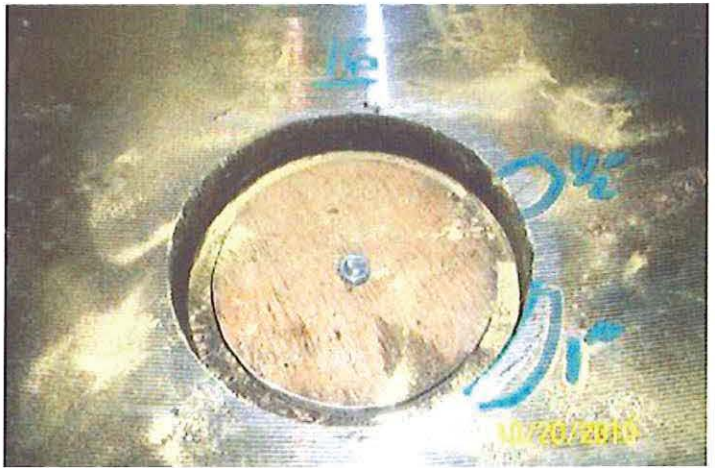
HOLE #16 WITH 1/2" & 1" LINEAR INDICATION AROUND HOLE
