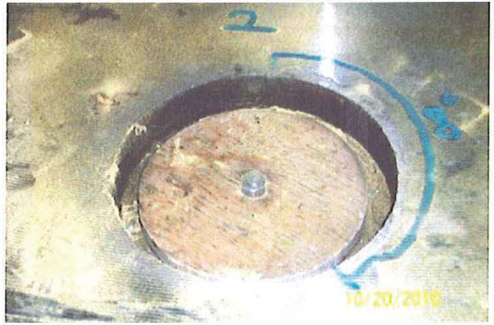
HOLE #2 WITH 8" LINEAR INDICATION AROUND HOLE
