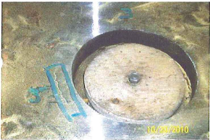
HOLE #3 WITH 5" LINEAR INDICATION AROUND HOLE
