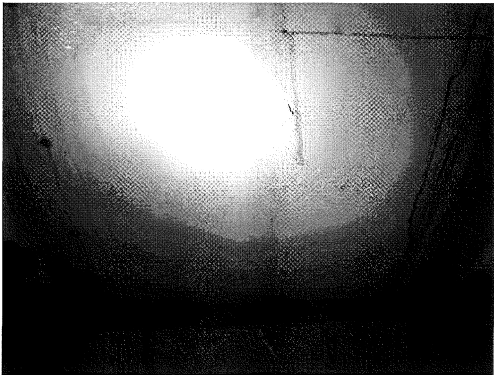
Figure 6 - Photograph showing the area of Valve 1 that was selected to be polished and have Replicas made.
