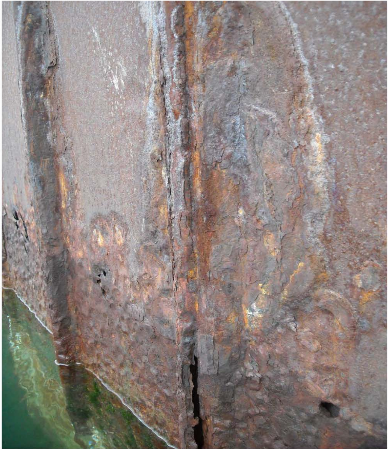
SSP Knuckles in Poor Condition (Open)
