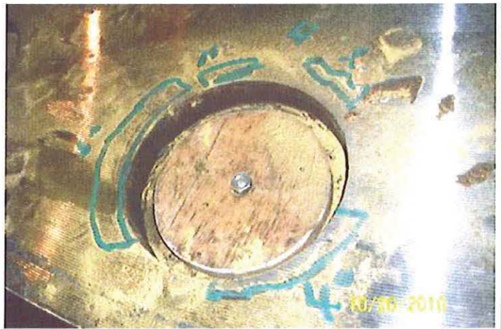
HOLE #4 WITH 7", 1", 2" & 4" LINEAR INDICATION AROUND HOLE
