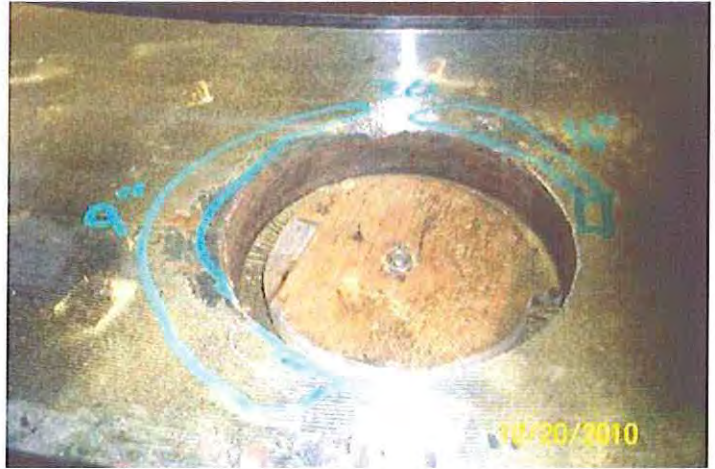
HOLE #19 WITH 9" & 4" LINEAR INDICATION AROUND HOLE
