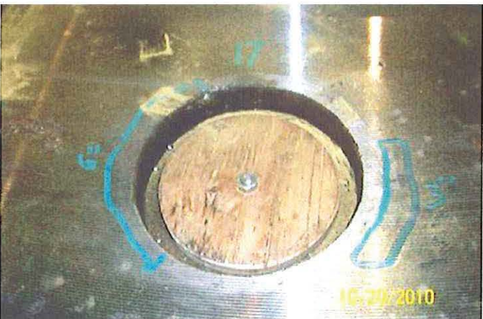
HOLE #17 WITH 6" & 3" LINEAR INDICATION AROUND HOLE
