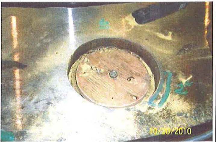
HOLE #6 WITH 2" LINEAR INDICATION AROUND HOLE
