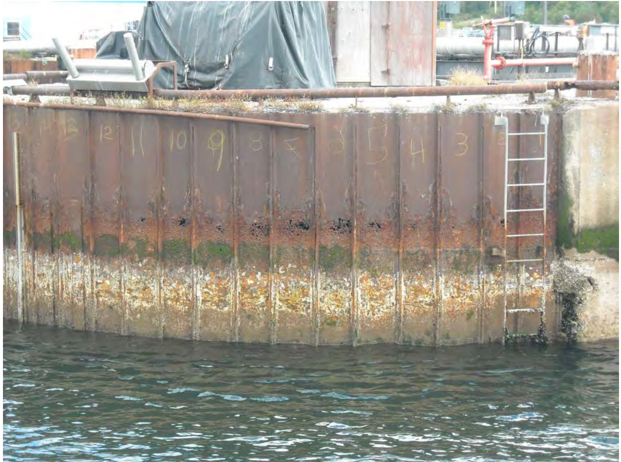
Typical SSP Condition in Tidal Zone Picture Taken at Low Tide (North Cell)
