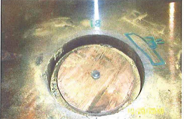
HOLE #18 WITH 3" LINEAR INDICATION AROUND HOLE
