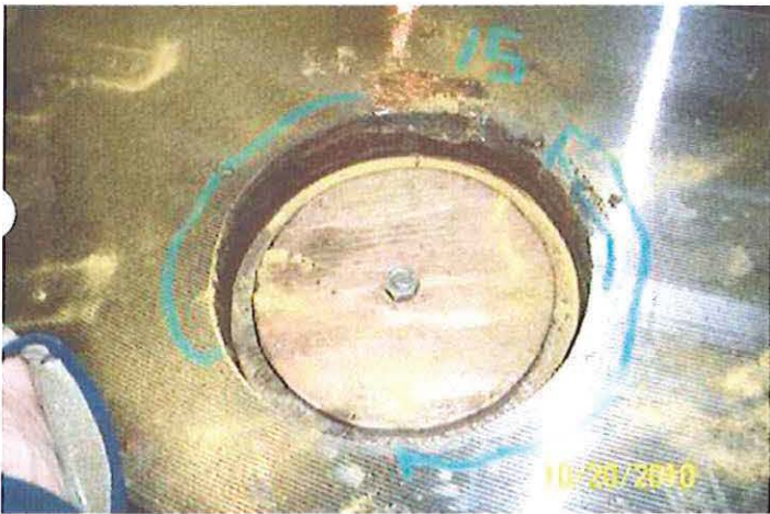
HOLE #15 WITH LINEAR INDICATION 60% AROUND HOLE
