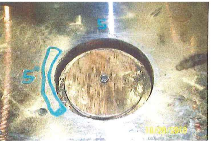
HOLE #5 WITH 5" LINEAR INDICATION AROUND HOLE
