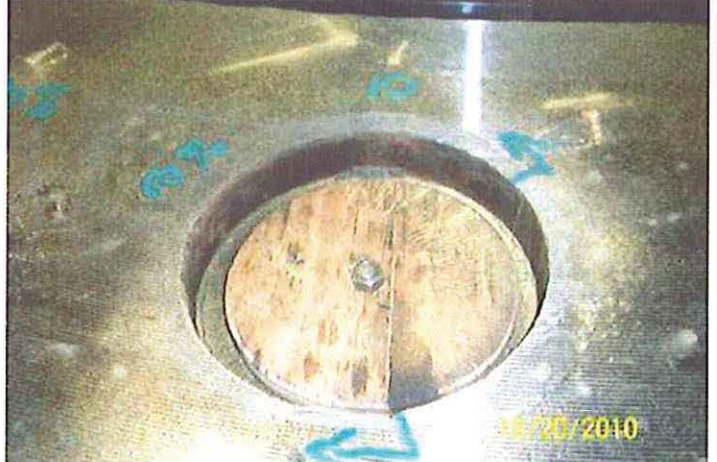
HOLE #10 WITH LINEAR INDICATION 60% AROUND HOLE
