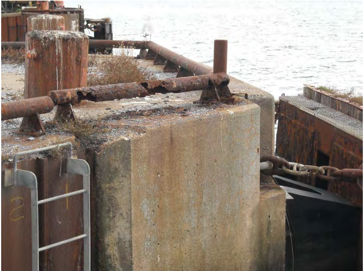
Safety Rail in Poor Condition
